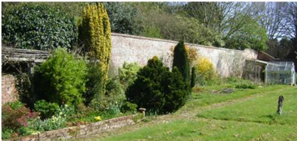
Photo shows the side perimeter of the original old wall of the kitchen garden (grape vine on the left). The wall extends along the back perimeter into the adjoining properties. Photo taken April 2015
